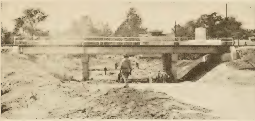
AN UNDERPASS UNDER CONSTRUCTION IN BOWIE COUNTY, TEX. THE PUMP HOUSE IS UNDER THE LEFT SPAN.
